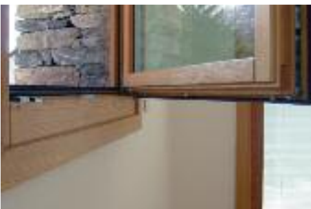
32_Carrello e fungo antieffrazione
